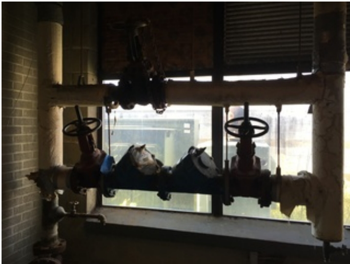
BFP branch water supply
