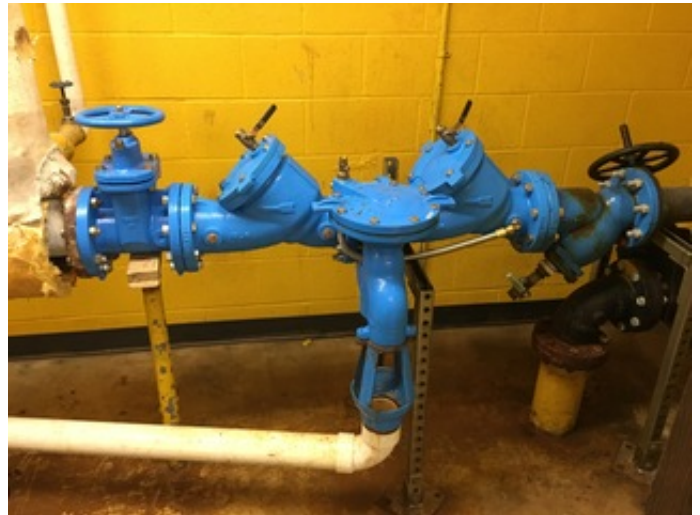
Main water BFP
