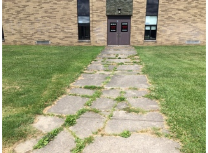
Rear east courtyard walk damage
