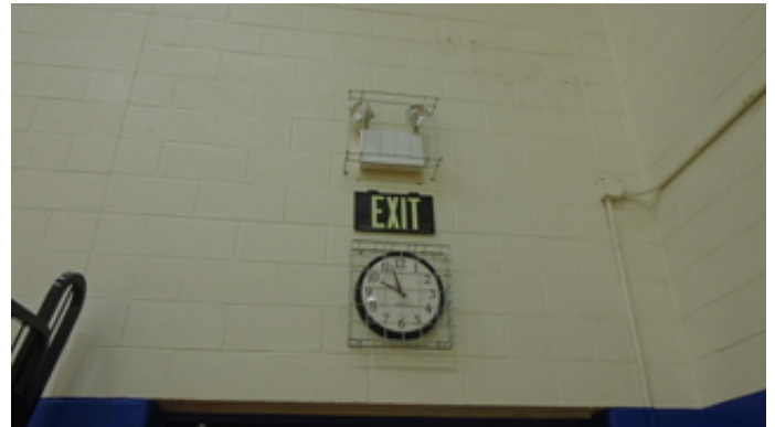
West House Gym Emergency Light and Exit Sign
