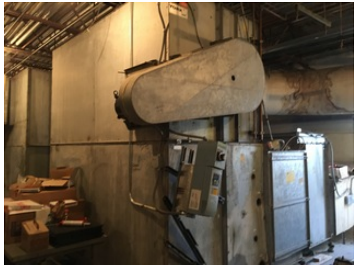
Air handling unit
