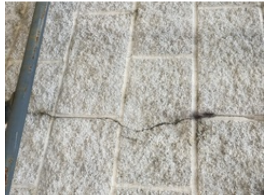
Crack at retaining wall
