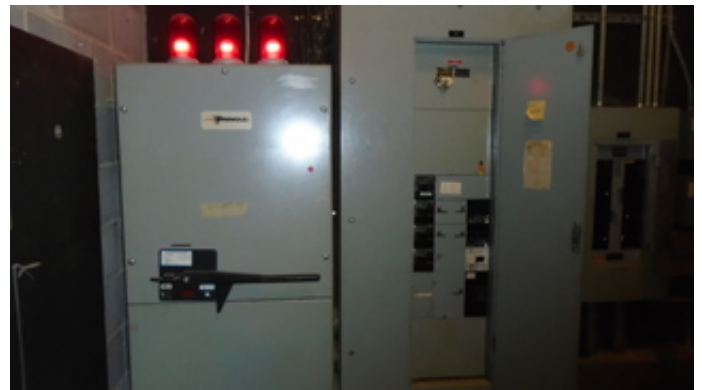
Electrical switchgear (West House)
