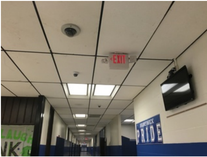
Ceiling mounted cameras
