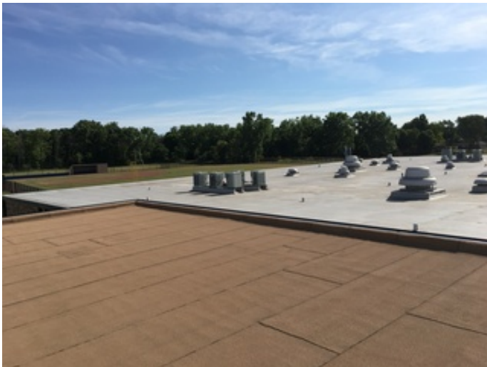
Roof mounted condensing units
