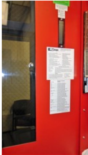
Fire alarm control panel
