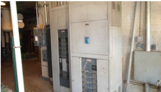
Electrical switchgear (East House)
