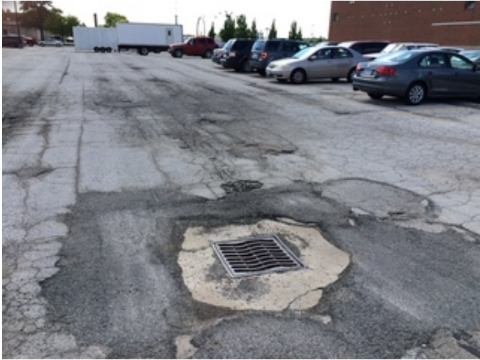
Front/west lot pavement damage
