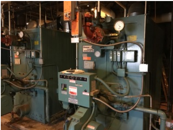
Heating water boilers
